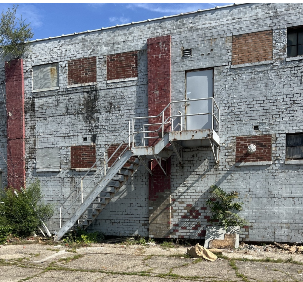
Windows up by the fire escape bricked up
